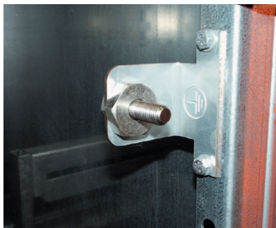
Pic. 9: Ground terminal studs
