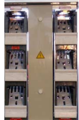
Pic. 8: Busbar insulating cover
