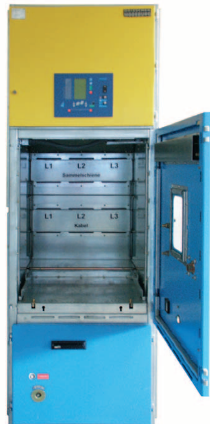
Picture 8: Open circuit-breaker panel type E3K with 3 chamber compartment without circuit-breaker
