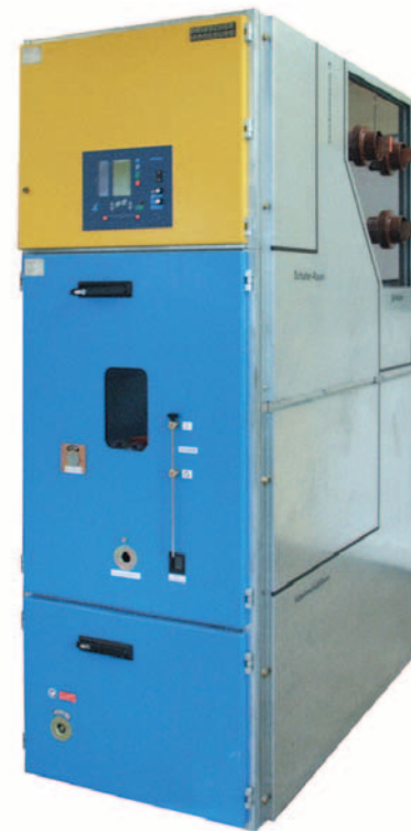
Fig. 4: Circuit-breaker panel with 3-compartment design type E3K
