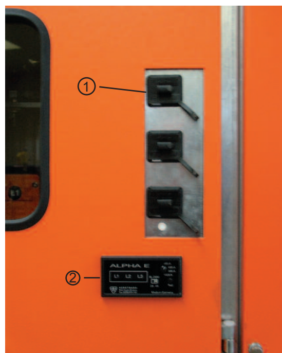
Picture: D-panel with capacitive interface and short-circuit indicator
