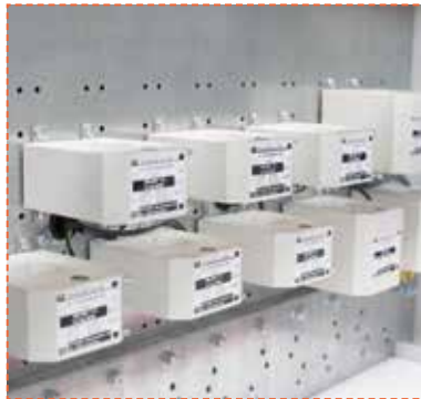
Current transformer installation
