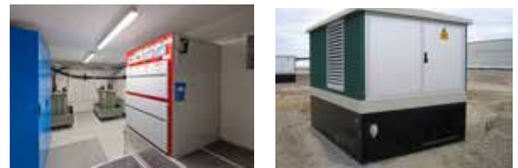
Fig. left: ECOS-Z shown in a walk-in substation, Fig. right: non-walk-in substation
