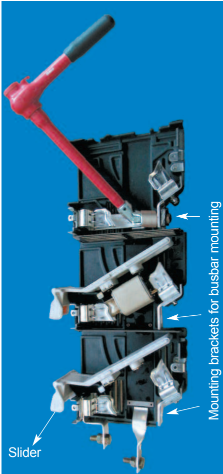
Pic 3: 403 system mounting situation on the busbar
